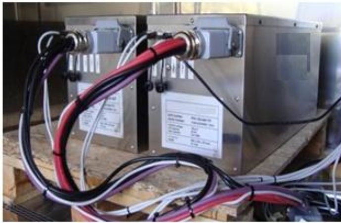
Fig. 1: Type B battery system under test
